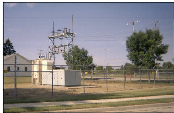
Substation in the Village of Black Creek
